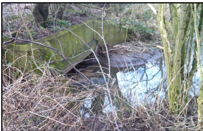
A silted box culvert
