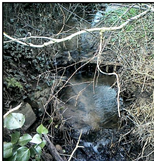
A partially obstructed trash screen
